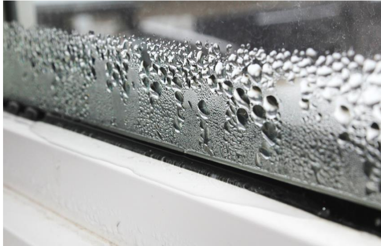
Fig. 27 Moisture condensation on external glass pane of the insulating glass unit
