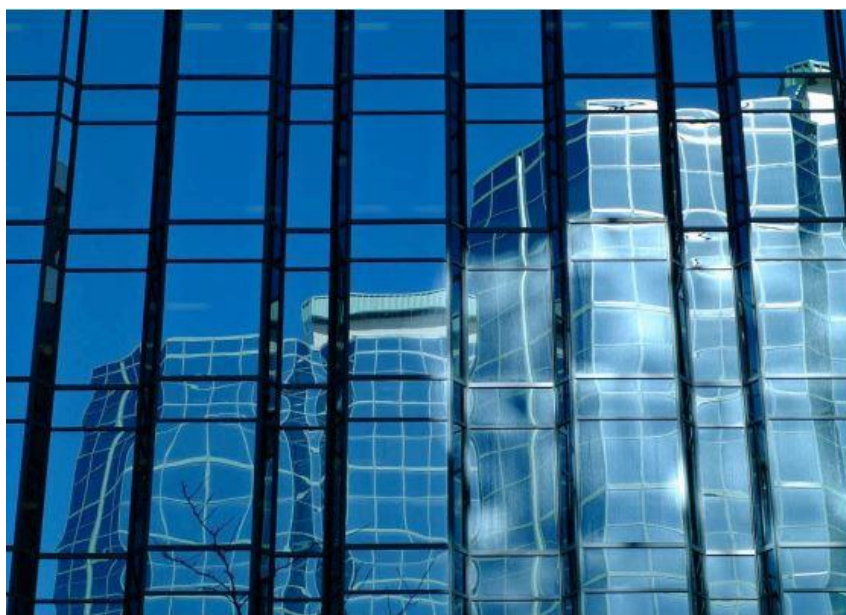
Fig. 29 Distortion effect, depending on concavity/convexity of glass panes due to overall bow and roller wave of toughened glasses, etc.
