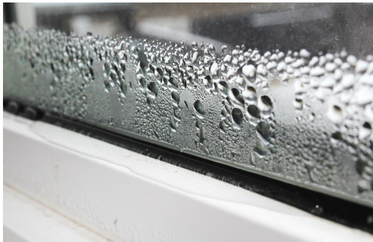
Fig. 30 Moisture condensation on external glass pane of the insulating glass unit
